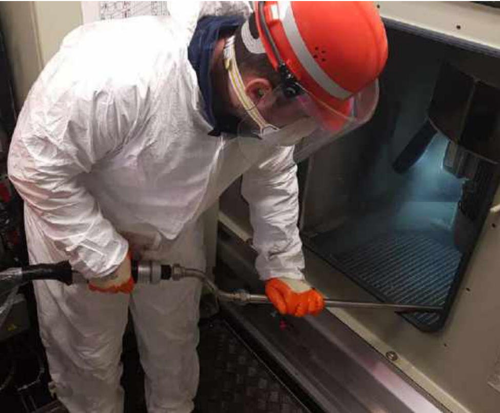
Cleaning of traction cooler
